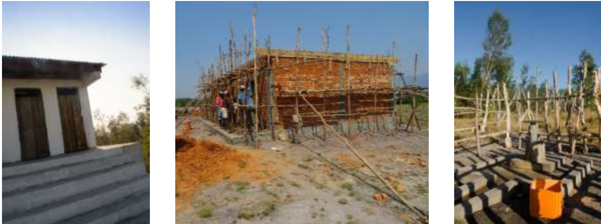
SEED's Module 1 construction activities at Manambaro Lycée including the first latrine block (left), the first new school building (centre) and the surface of the 21 metre deep well (right)
