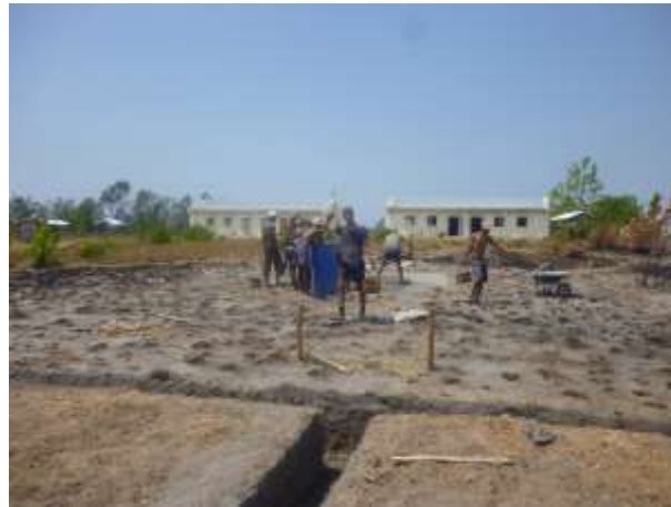
Manambaro Lycée’s original school building in the background as work begins on the first new school building
