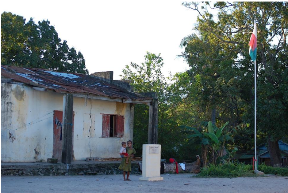
The crumbling state of schools in the Anosy region
