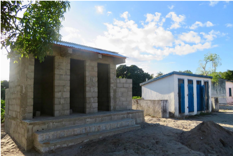
New latrine blocks being built in a previous phase of Project Sekoly, next to the school's existing aging infrastructure
