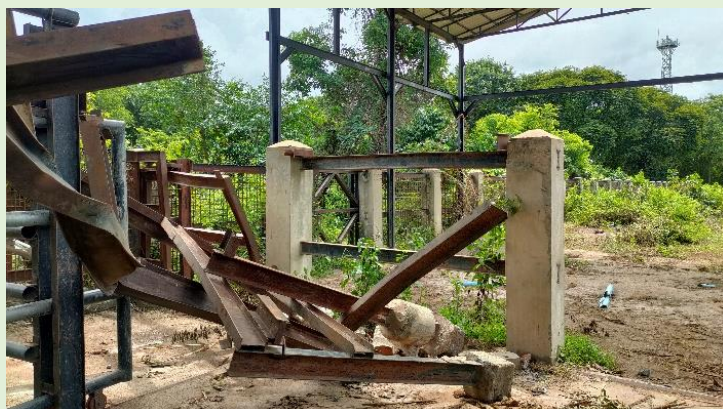
Damage to elephant enclosure caused by Sakor
