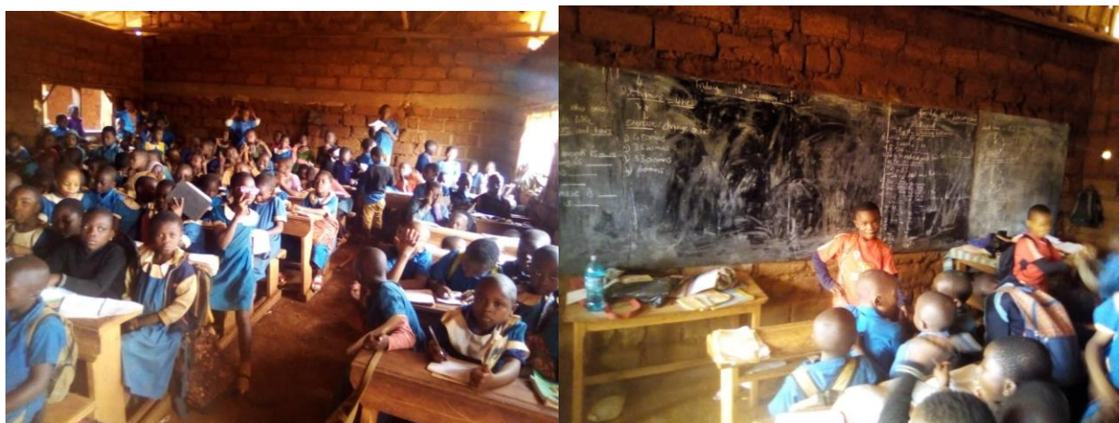
Floor of classroom not cemented and walls not plastered
