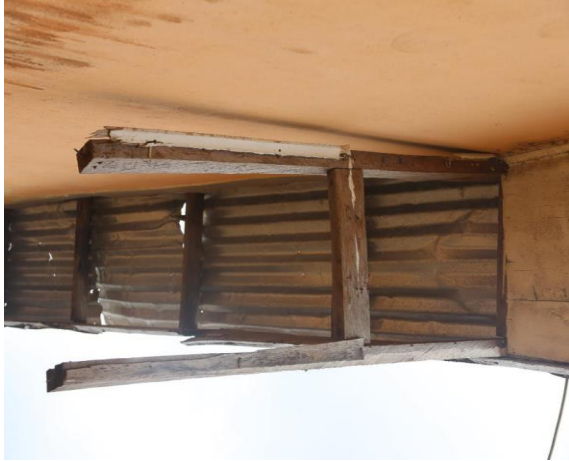
Zinc of one classroom falling off because off as a result of rough winds
