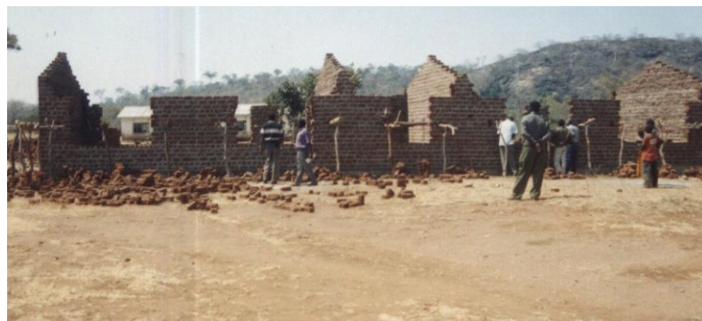
A COMMUNITY SCHOOL UNDER CONSTRUCTION AT NYEMBE VILLAGE IN CHIEF BANGOMBE'S AREA,
