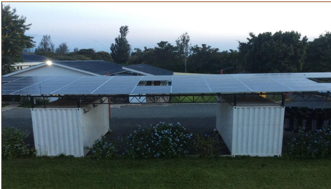
Kivulini Maternity Centre solar electricity panels
