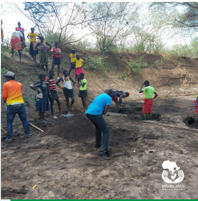
Figure 1: Pegging and marking process of the foundation trench for guidance before excavation started,
