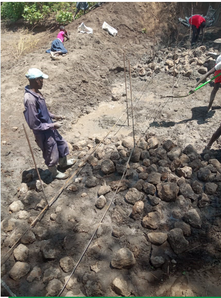
Figure 5: Portion of dam reinforced by Y-20 and Y-10 bars, barbed wire used for linkage of bars.
