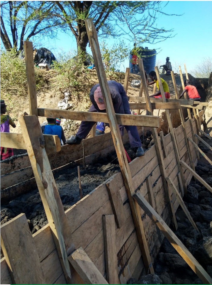
Figure 6: Placing of form work attaining the shape of the dam, just immediately after finishing the slab
