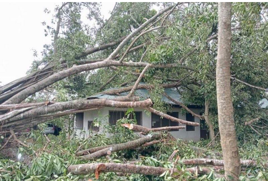
Dormitory and kitchen: After the typhoon
