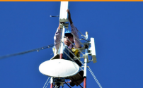
PHOTO: INSTALLATION OF APPLIANCES IN THE MAIN TOWERS BY A FILANTHROPIST FELLOW
