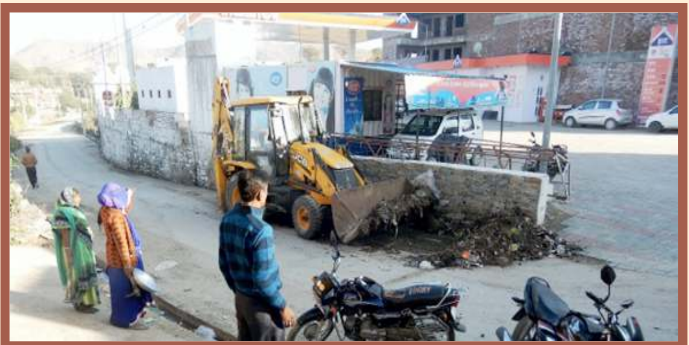
Figure 4: Legacy waste being removed by Seva Mandir before starting awareness on NOW
