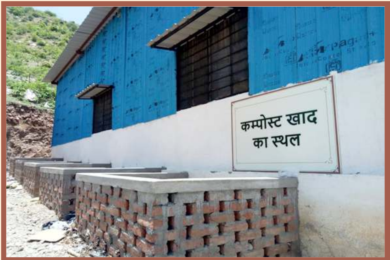
Figure 33: NADEP compost pits for wet waste composting
