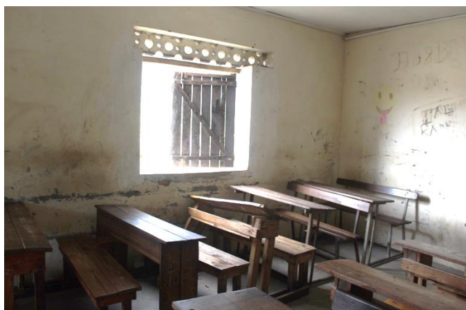
Broken benches at a lower secondary school.
