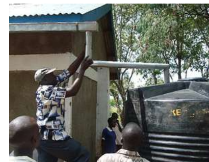
Water collection system
