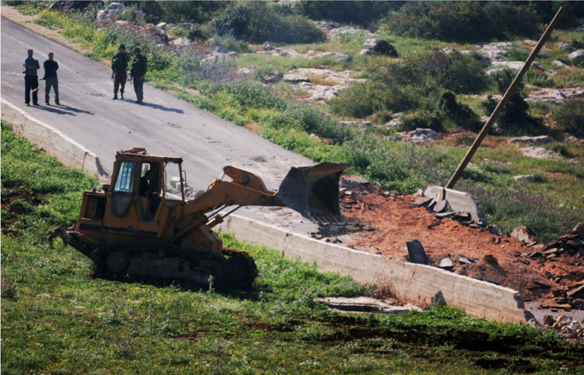
April 7, 2011: Israeli Army Demolition Bulldozers destroy Peace Road and two small homes with animal stables
