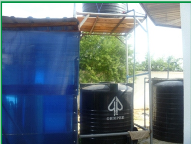
Borehole and Water Treatment
